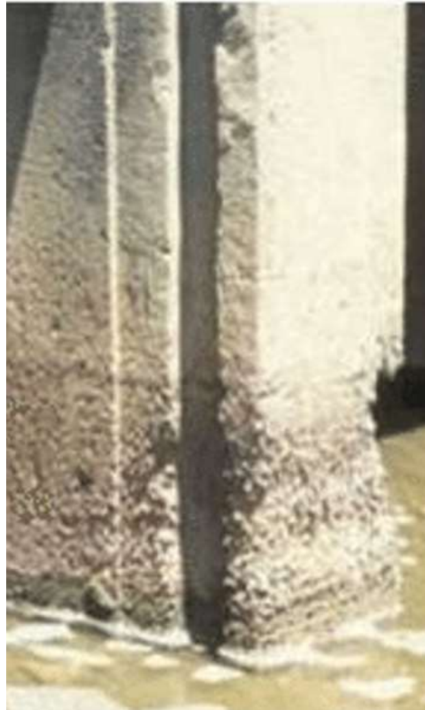
Sewage plant – Sulphate attack
